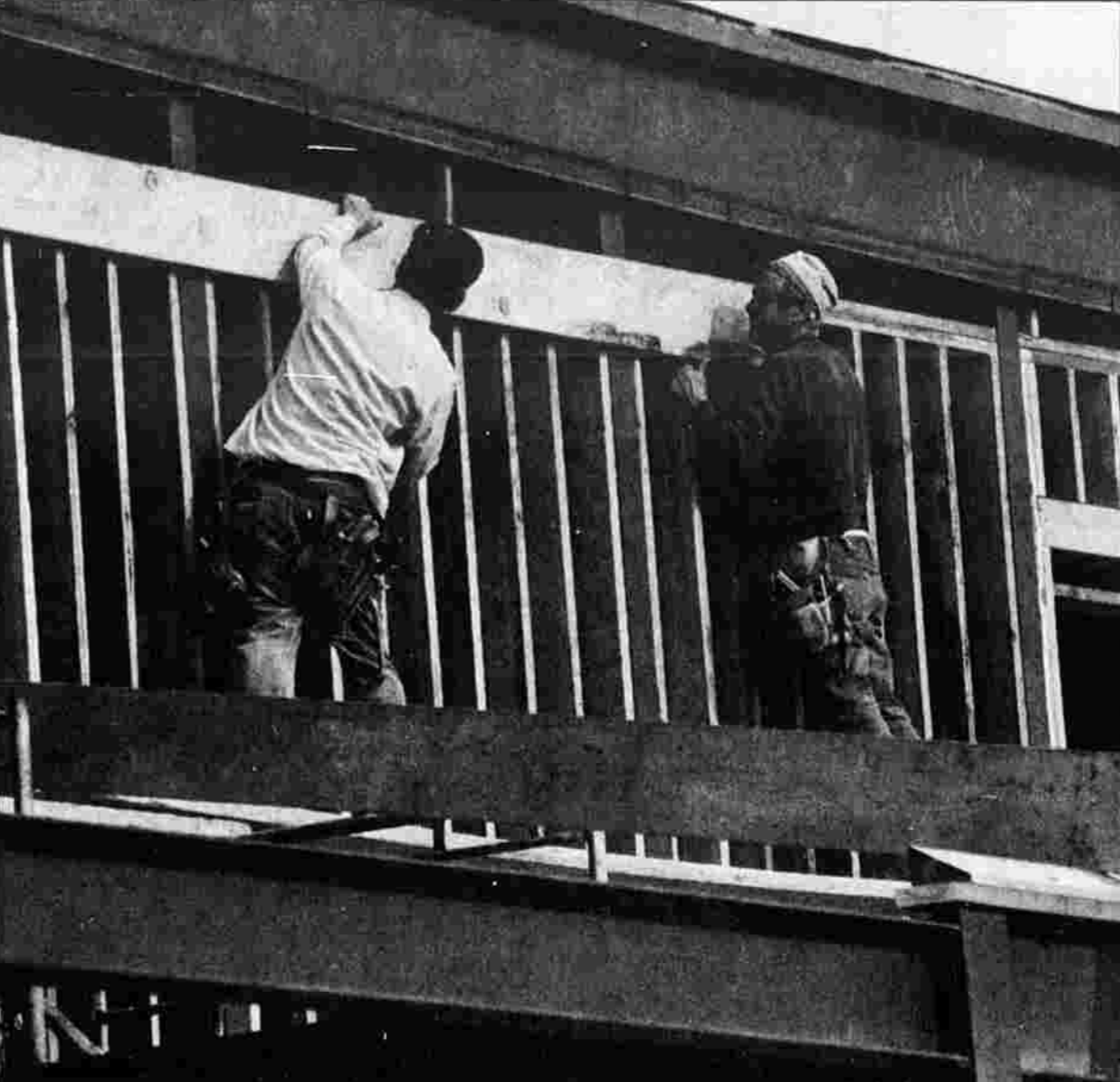
FRAMING A BUILDING — Jean-Yves Couture, left, and Ray Sirdis of CCL Construction Corp., put up the frame for the new post office building on Sheldon Road in Manchester.
